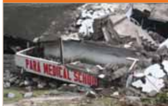
PARAMEDICAL SCHOOL DESTROYED BY THE EARTHQUAKE IN PAKISTAN
